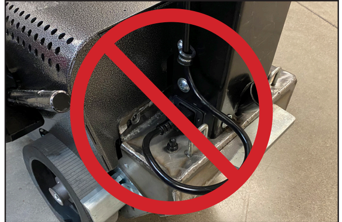
Power cord should NOT have excess slack.
